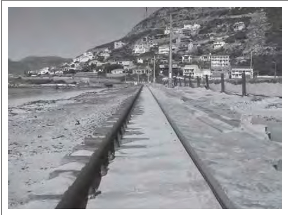
Figure 9.1: Exposure of the Glencairn Rail to coastal processes such as wind-blown sand Photograph: D. Colenbrander
