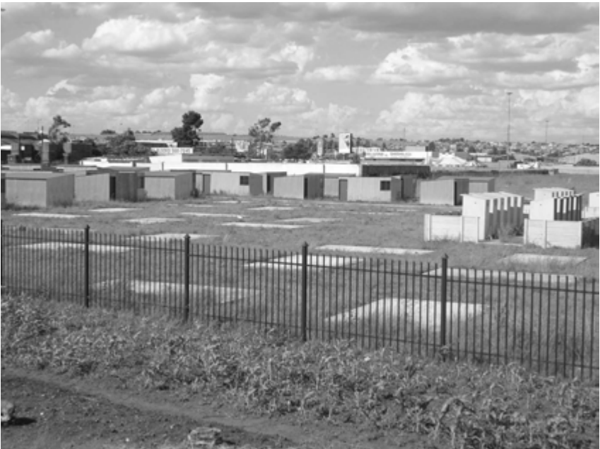
Figure 5.5: The Protea South temporary relocation area under construction on state-rented, privately owned land in 2006 (top); unused and being dismantled in 2009 (bottom)
